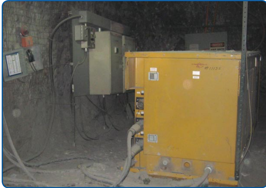
Figure 1: Telephone Station in Underground Mine
