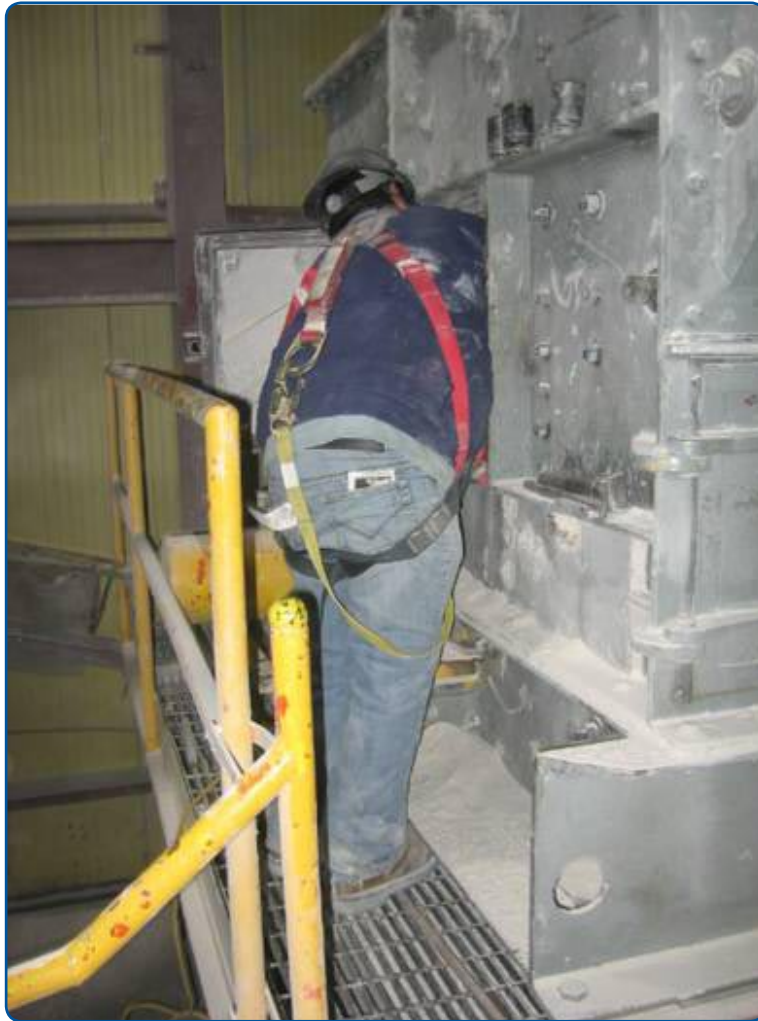
Figure 1: Crusher Maintenance. Note: worker is wearing a belt with harness and has a quick reference safety checklist in his back pocket
